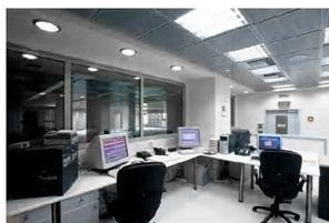
Network Operation Center
